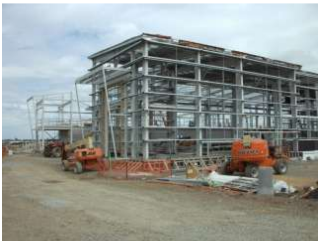
Figure 1: View south with floor pits in the foreground and southern steelwork in the background
