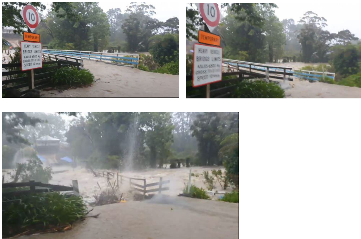
Figure 3 – Impact of flooding on the bridge
