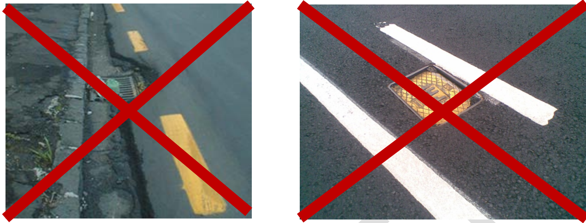
Figure 82: Examples of maintenance issues,, creating hazards to cyclists - through high asphalt lips at road edge (left) and sunken cover (right)
