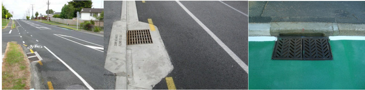
Figure 83: Cycle lane with acceptable grate and lip-less road surface (left to right: Triangle Rd, Ian McKinnon Drive, example from Sydney)
