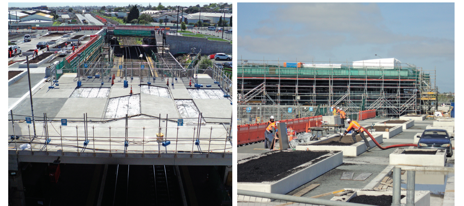
Construction continues on the new pedestrian plaza which will connect both station platforms and the new Panmure Station Road
