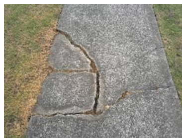
Footpath – crack broken
