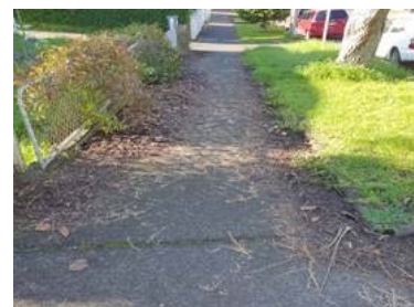
Footpath – vegetation and slippery
