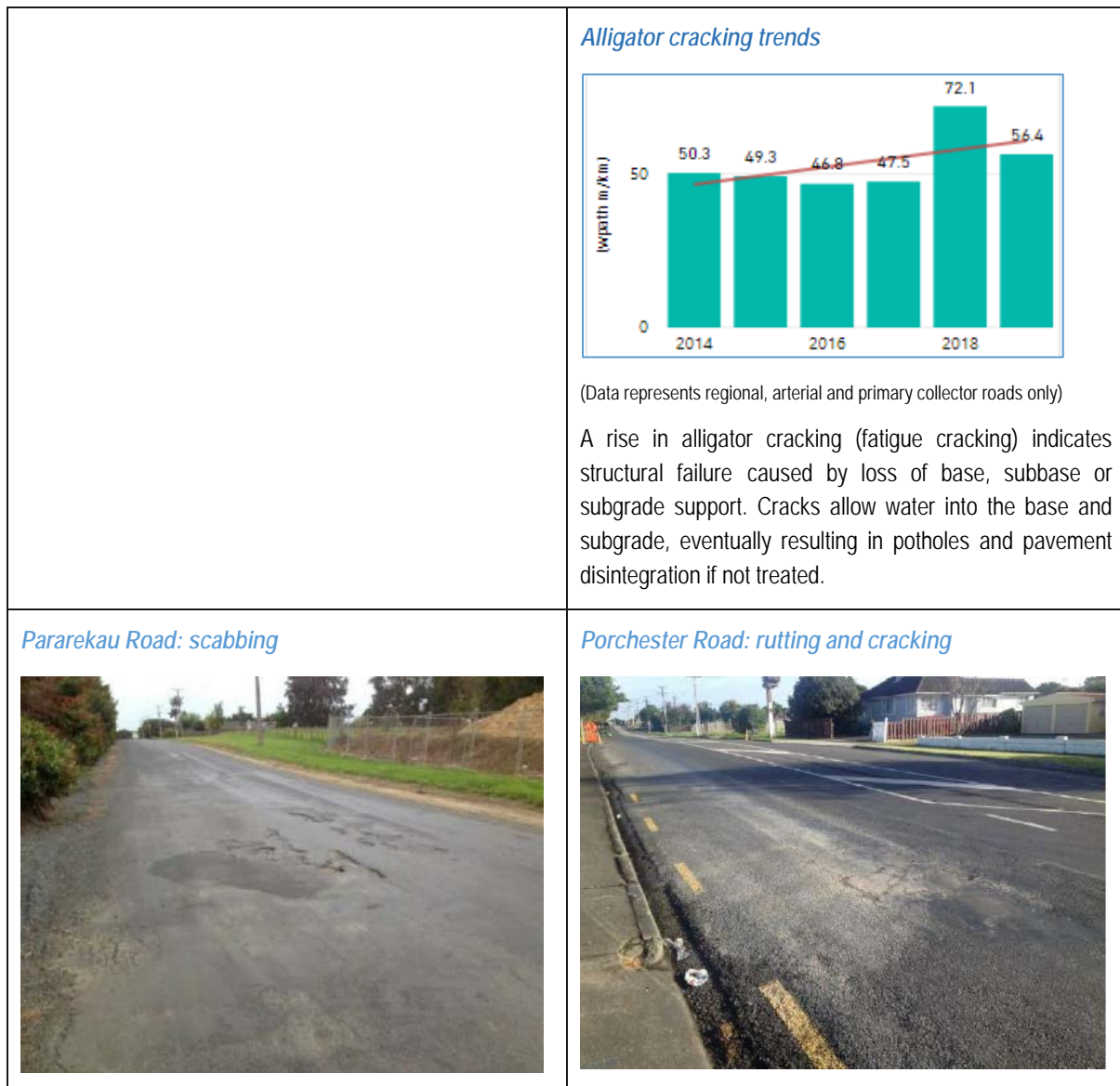
Figure 7-1: Sealed roads – evidence of asset deterioration
