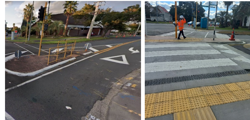
Before and after photos of the pedestrian amenity at the Buscomb Avenue leg of the intersection
