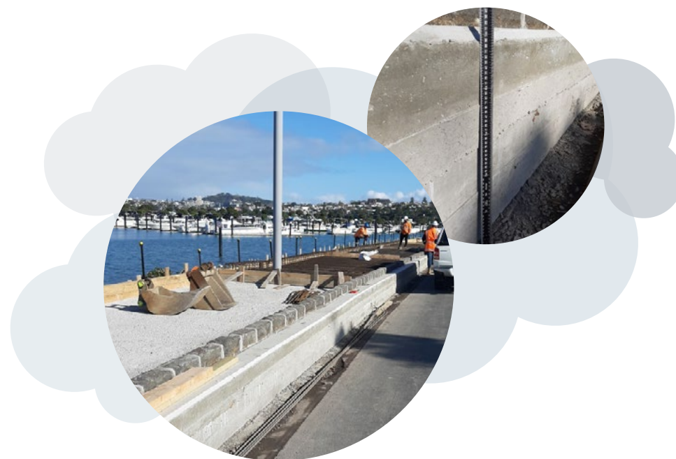
FIGURE 10: AT HAS RAISED THE HEIGHT OF THE TĀMAKI DRIVE SEAWALL TO IMPROVE RESILIENCE TO SEA LEVEL RISE
