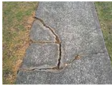
Footpath – crack broken
