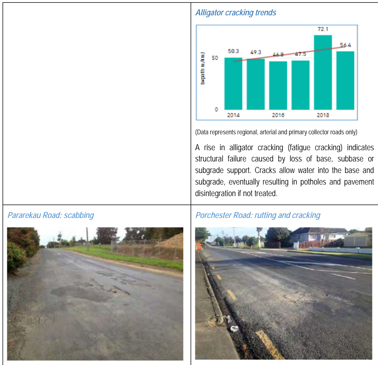
Figure 7-1: Sealed roads – evidence of asset deterioration
