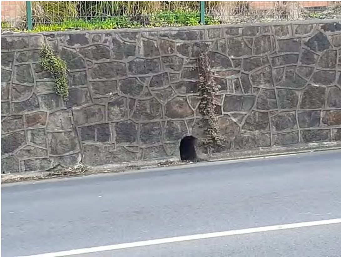
Observation # 7, photo 2 - One large void looks formed may be drainage
