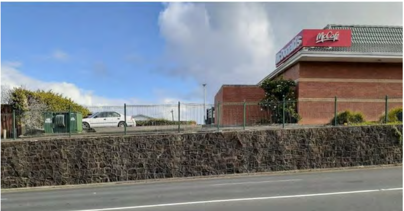
Photo 2-1: Retaining Wall along the western edge of Lake Road between Roberts Road and Bayswater Avenue
