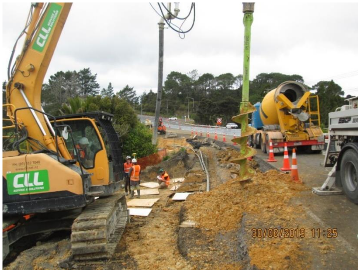
Work on retaining structures at Dairy Flat Highway intersection with Coatesville Riverhead Highway
