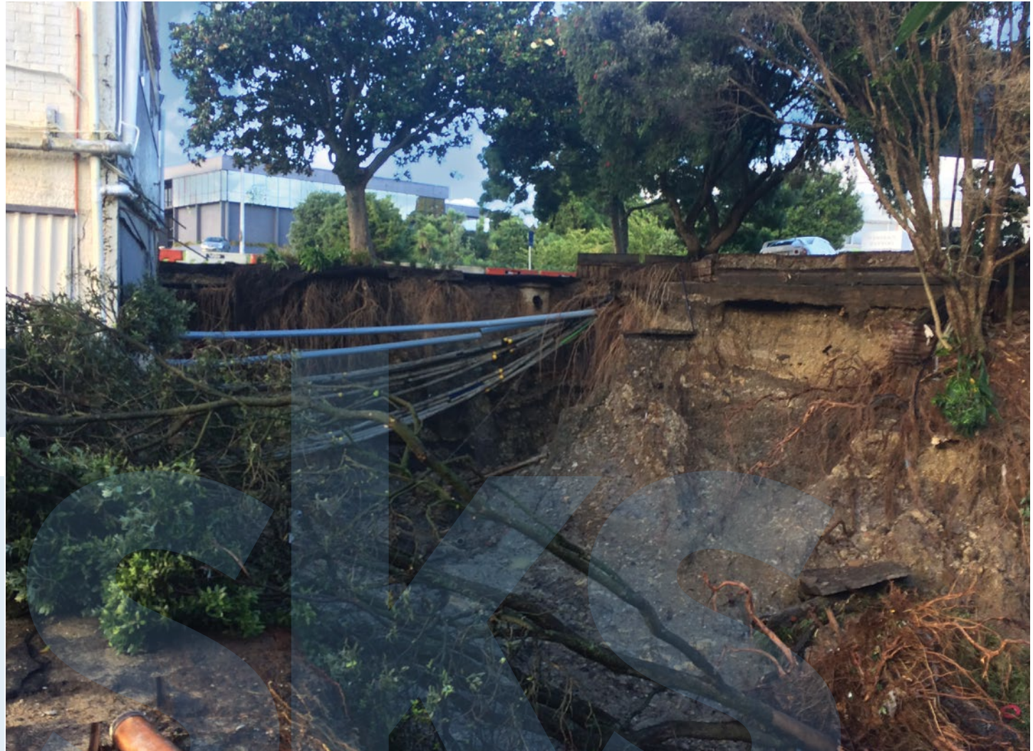
CLOSURE OF GREAT NORTH RD, NEW LYNN, JUNE 2017. INTENSIFICATION MEANS MORE STORMWATER RUNOFF, AND EXTREME WEATHER EVENTS ARE BECOMING MORE COMMON DUE TO CLIMATE CHANGE
