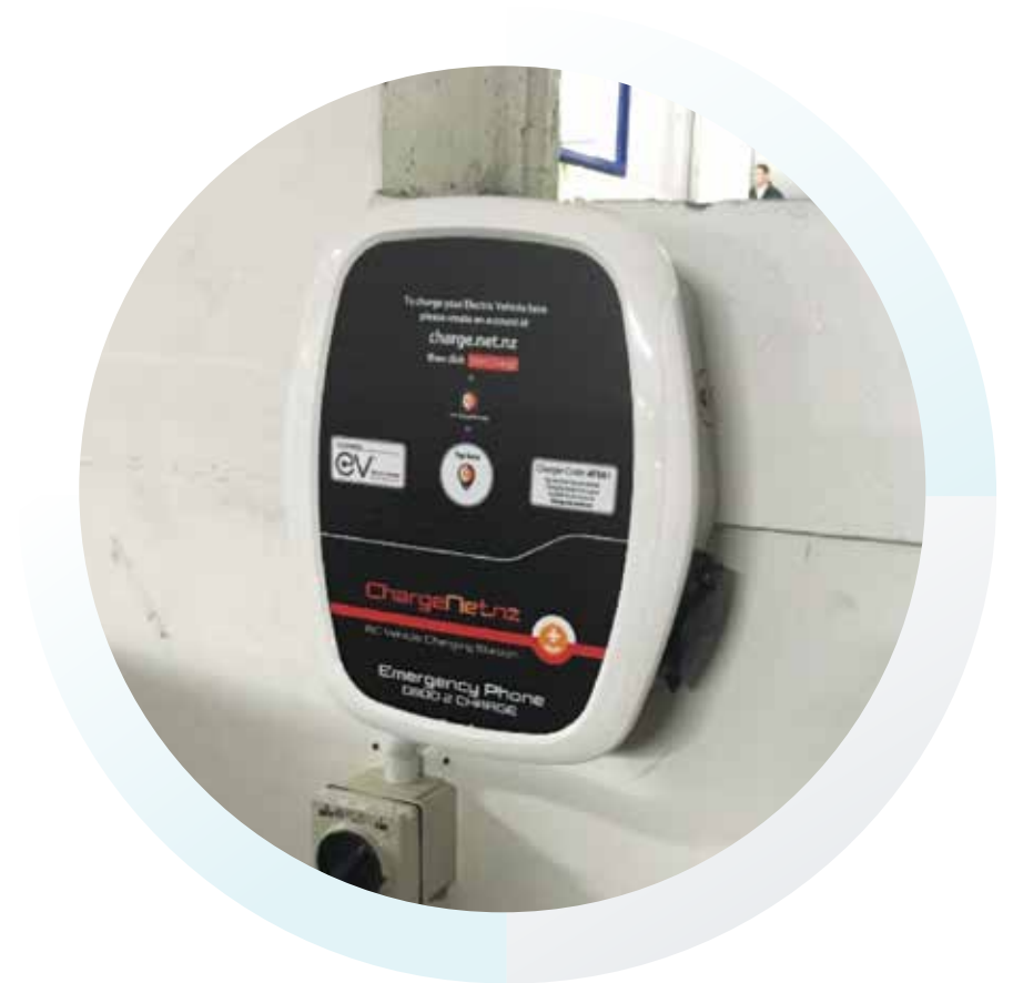
An example of a charger installed in Downtown Carpark.
