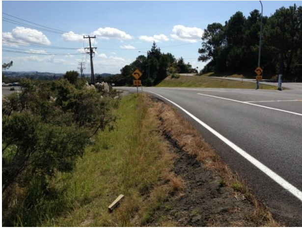
Before photo – non recoverable slope near Okura River Road where vehicles have left the road
