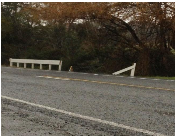
Before photo – wooden rail impacted by vehicle providing inadequate protection
