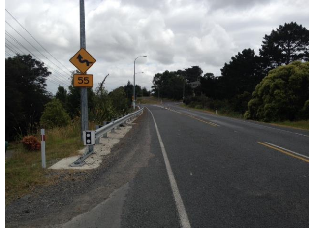
After photo – installation of guardrail near Okura River Road to protect non recoverable slope
